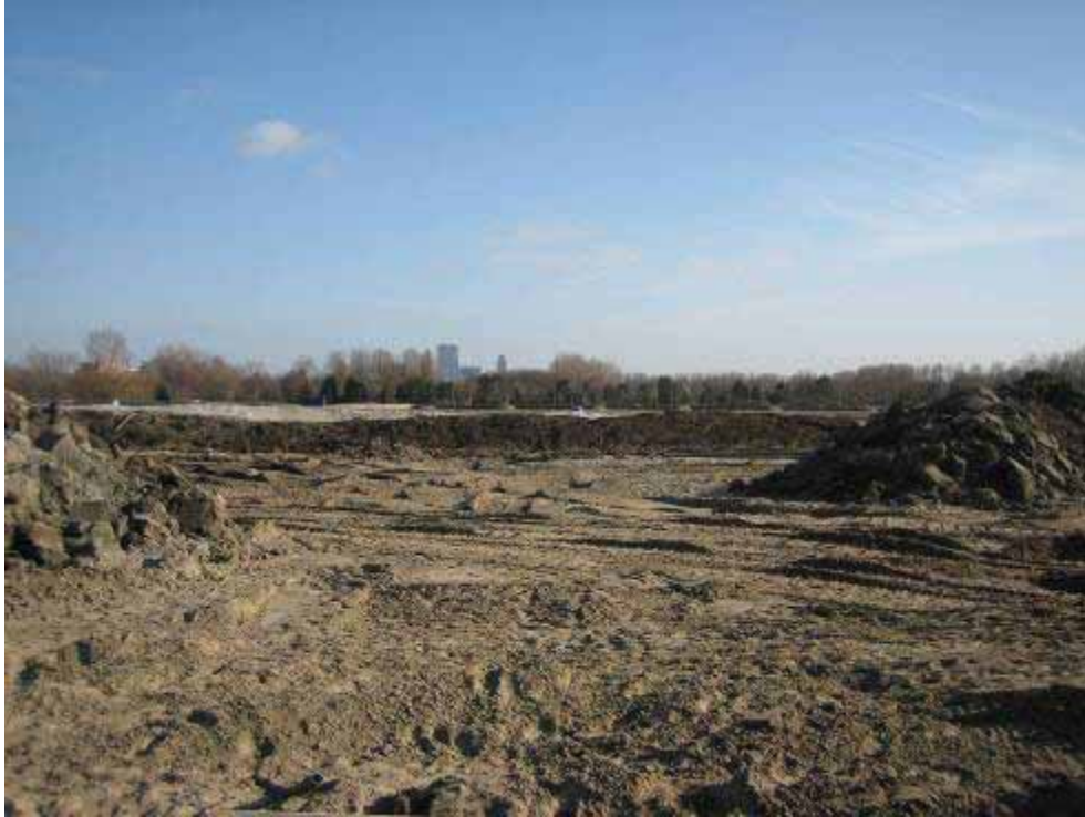
Picture 6.11 Zestienhoven under construction, building-site preparation activities consist of moving around a whole lot of soil Source: Author
