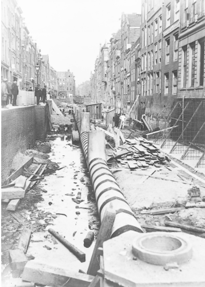
Picture 4.18 Construction of the sewer in the inner city around 1870. Source: Municipal Archive Rotterdam
