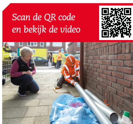
Figure 4: Stadsbeek project newsletter highlighting the decoupling of rainwater pipes by homeowners.
